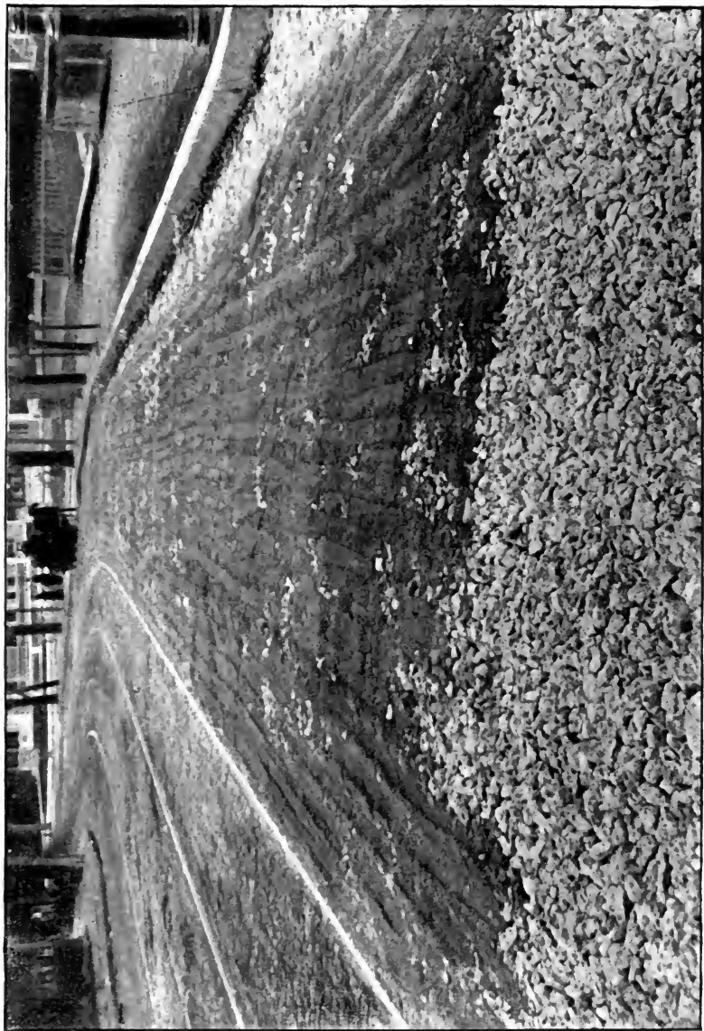
Warren St., Boston, 1892. Repairs on a macadam road; showing method of binding and rolling.
